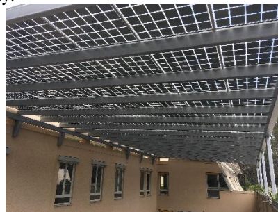
Figure 7 : Canopy on ADEME building – 2ES company – 26 kWc
