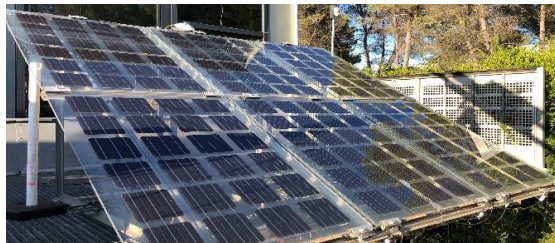
Figure 5 : Canopy mockup on CSTB plateformes – Onyx Solar® modules in BIPVBOOST project – 0,9 kWc.
