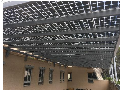
Figure 7 : Canopy on ADEME building – 2ES company – 26 kWc
