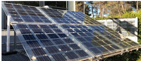
Figure 5 : Canopy mockup on CSTB plateformes – Onyx Solar® modules in BIPVBOOST project – 0,9 kWc.
