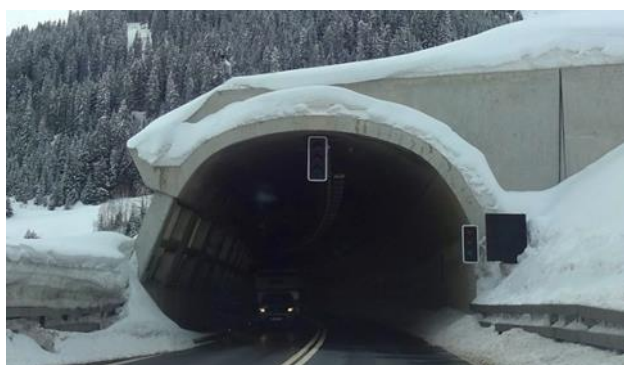
Figure 4. Entrance of the Cassanawald tunnel with portal collar in winter 2014, San Bernardino national highway. The width of the portal collar is 50 cm and the depth of the accumulated snow is about 80 cm.
