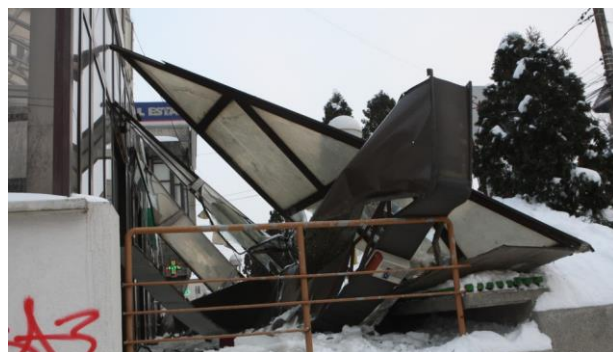
Figure 15. Collapse of a new metallic roof structure in Iasi [27]
