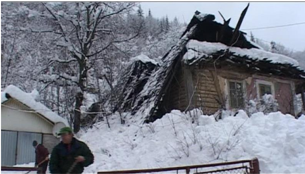
Figure 17. Collapse of a wooden roof structure in Cavnic [29]
