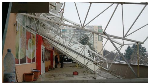
Figure 14. Collapse of a new metallic roof structure in Cluj [26]
