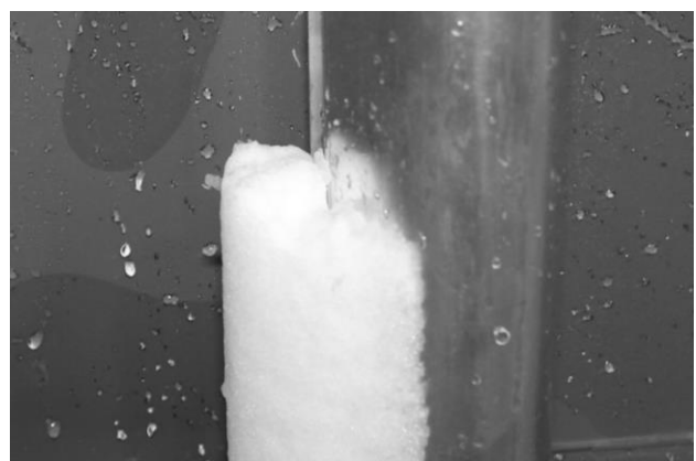
Figure 5. Example of wet snow accumulation (after partial shedding) on a mullion in a climatic chamber simulation.
