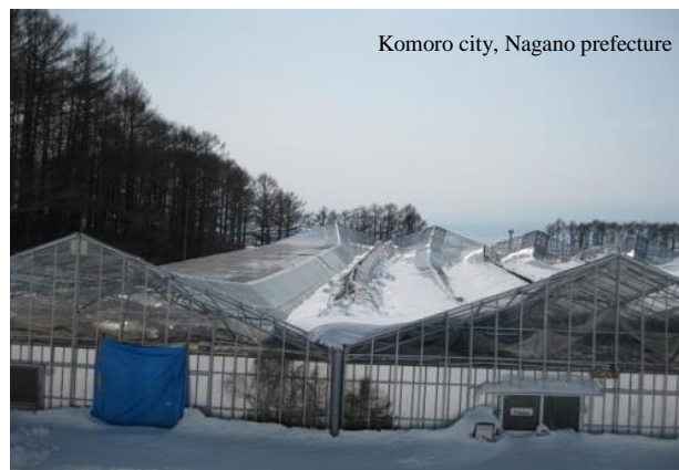
Fig. 2 Collapse of greenhouse due to excess snow load
