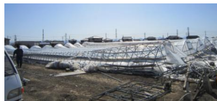
Figure 13. Collapse of a reinforced pipe-framed greenhouse due to snow load.
