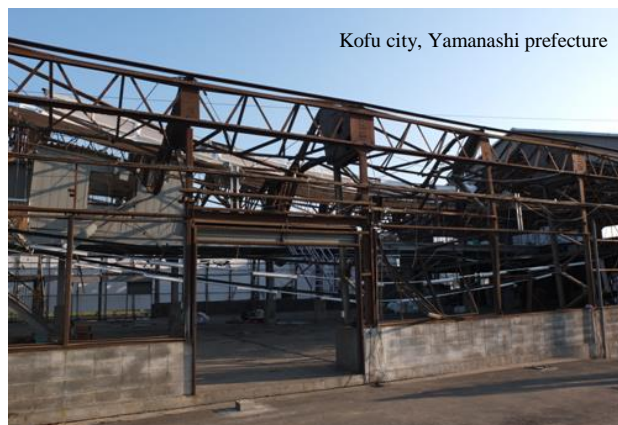
Fig. 1 Collapse of packhouse and equipment for packing
