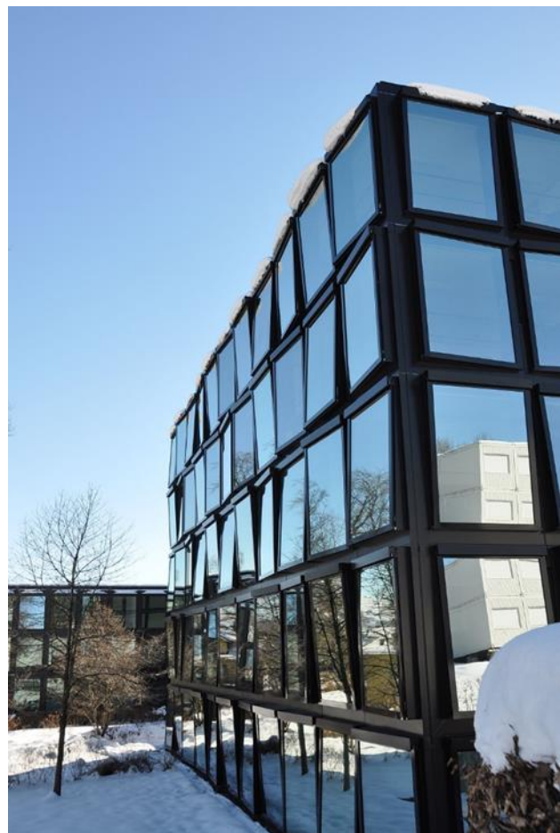
Figure 9. Snow accumulations on the window boxes of the existing Helvetia building on 10 February 2015.
