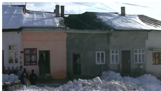
Figure 16. Collapse of an old wooden roof in Suceava [28]
