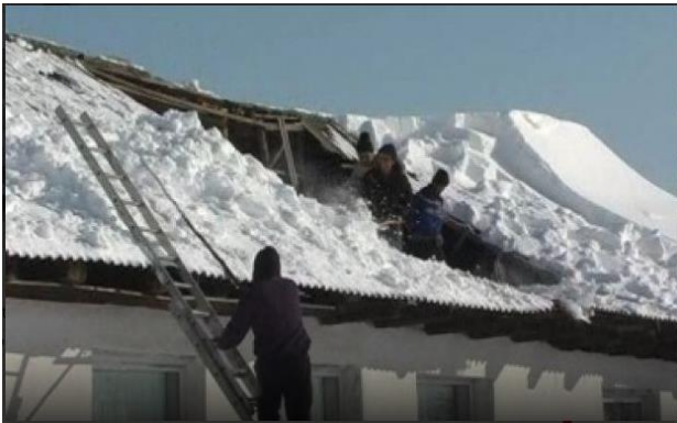
Figure 18. Collapse of a wooden roof structure in Podgoria [30]
