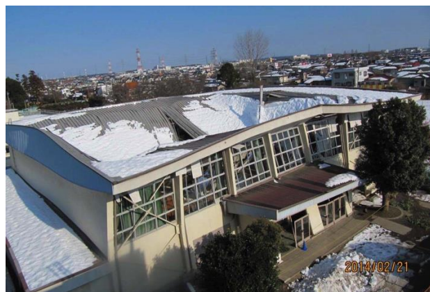
Photo 3. Example of collapsed building. (No.9 in Table 1.)
