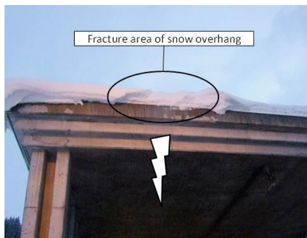
Figure 2. North entrance of the San Bernardino tunnel on 1 February 2014 with the fractured snow overhang (Photo Tiefbauamt Graubünden).
