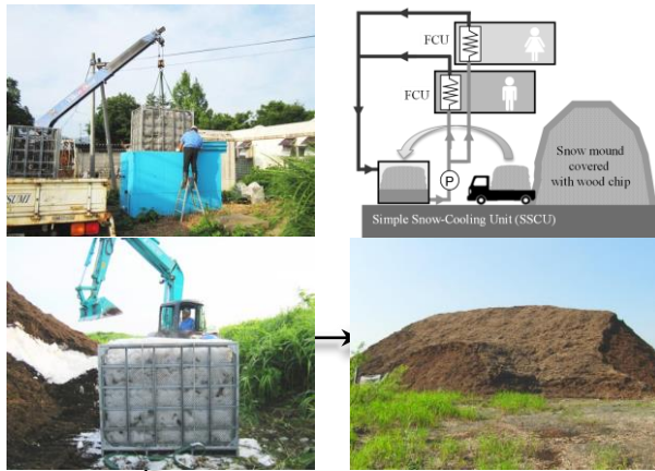
Figure 6. Snow cooling system for Highway SA lavatory.
