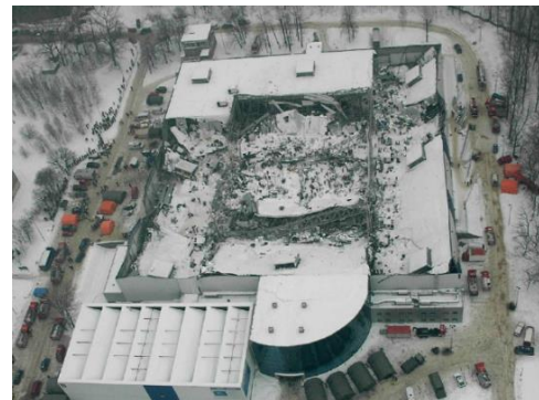
Figure 1. Roof collapse of Katowice Exhibition Hall
