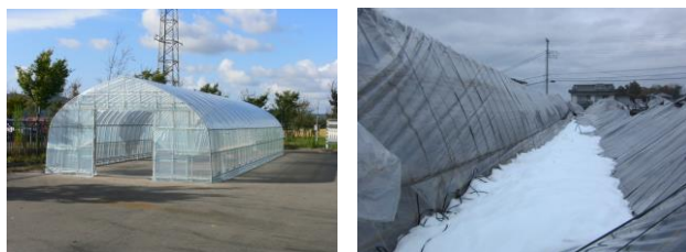
(a) Example (b) Collapse due to heavy snow Figure 1. Pipe-framed greenhouse.
