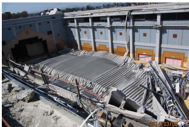
Photo 1. Example of collapsed building. (No.7 in Table 1.)
