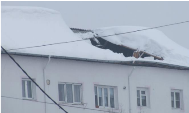
Figure 19. Collapse of a wooden roof structure in Focsani [31]
